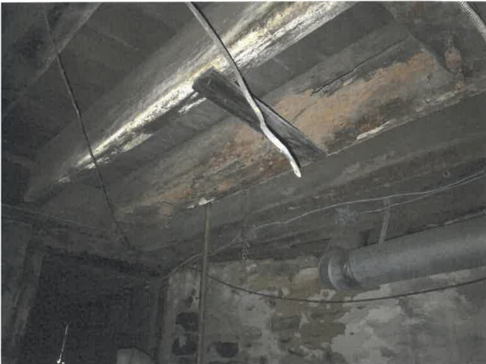
Moisture Decayed Floor Joists under Dining Room
