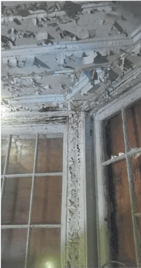
Damage at Bay Window
