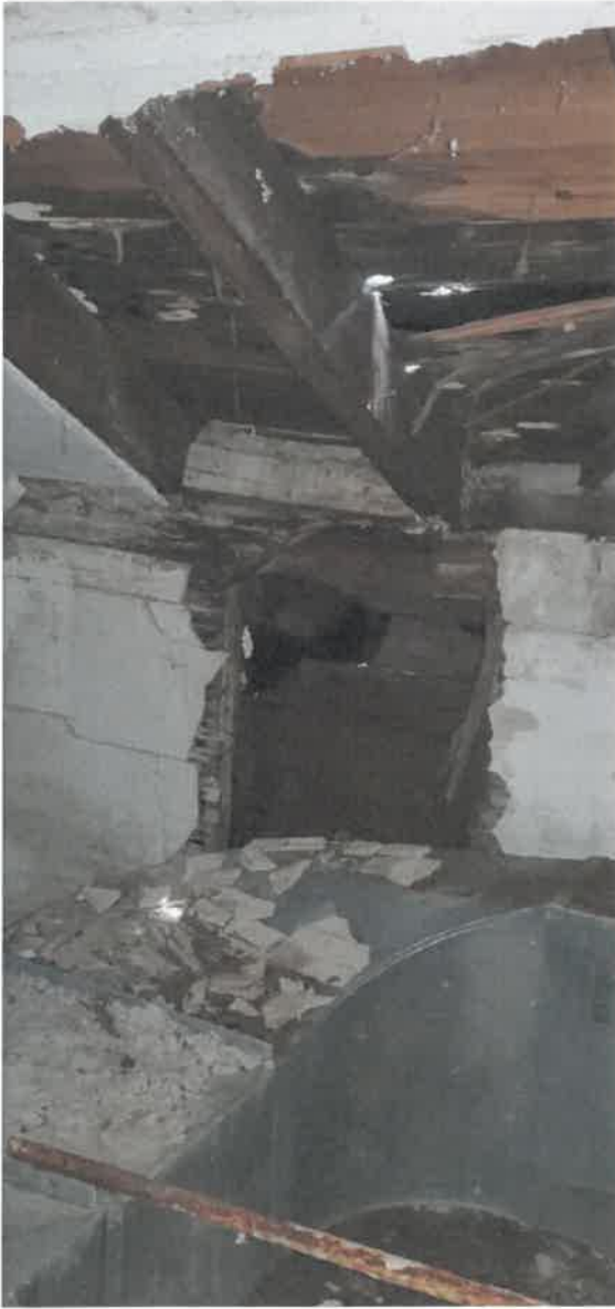
Damage Within Eaves
