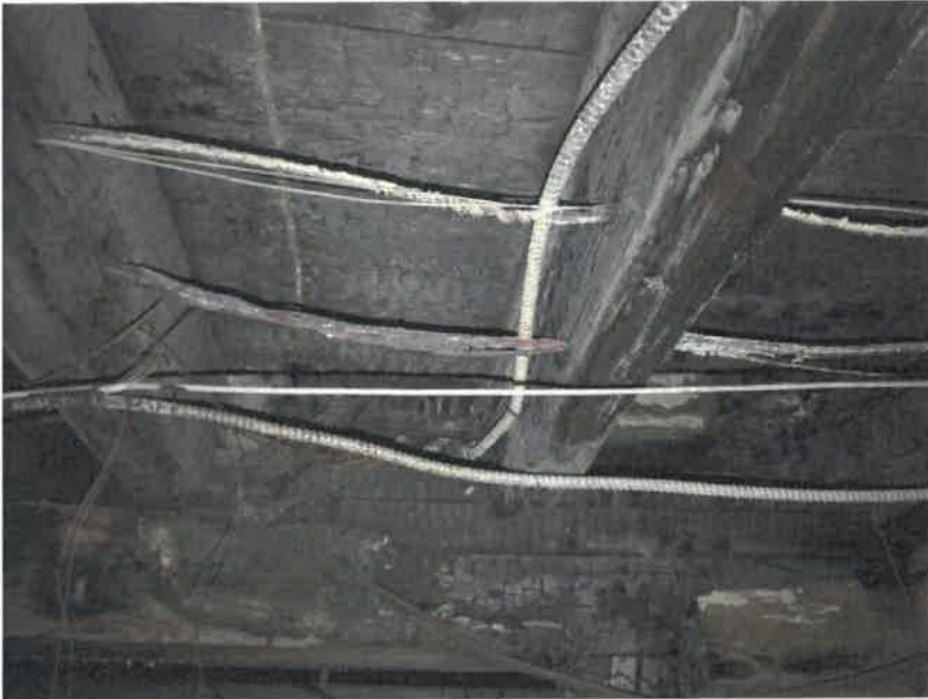
Fire Damaged Basement Floor Joists at Front Entry Hall
