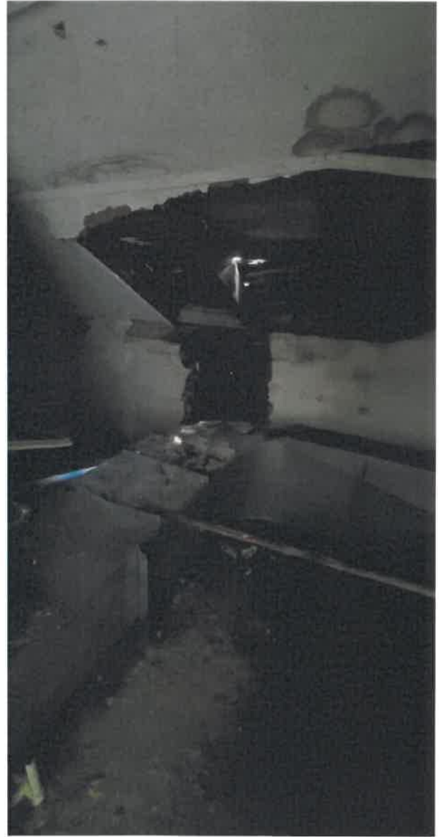
Damage Within Eaves
