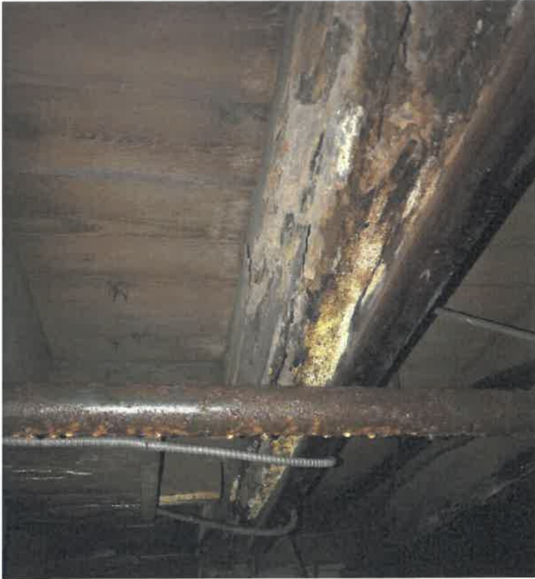
Moisture Decayed Floor Joists under Living Room
