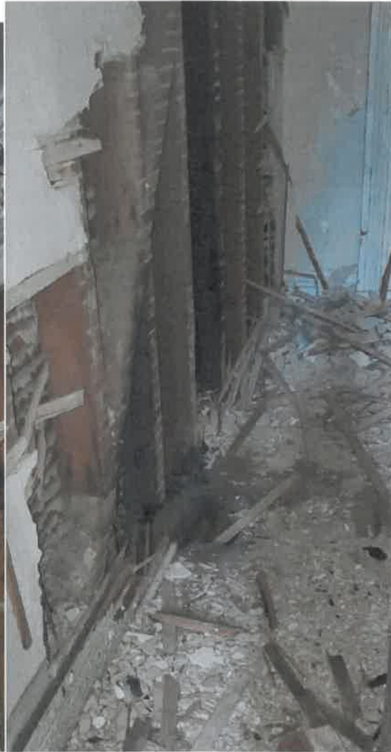
Front Entry Fire Damage
